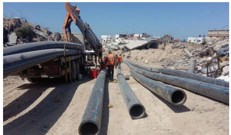
Repair of Bani Suheila water line by COGAT | Source: Jihad Land on Telegram, t.me/eretz
