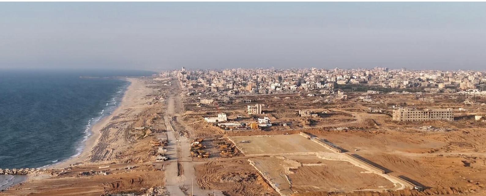
Construction of a new port in Gaza as part of a US-led project to bring aid into the Strip, via a floating pier | Source: Defense Ministry Department of Engineering and Construction
