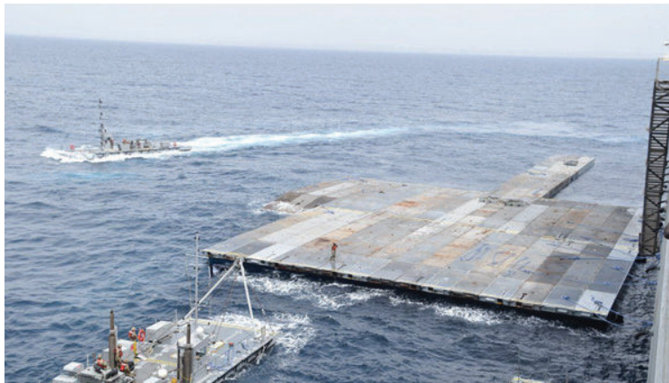
US Pier being built off the shore of Gaza | Source: US CENTCOM
